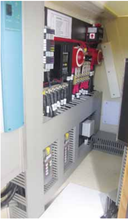
Power shut-offs, inverter and cable runs neatly recessed in saloon bulkhead. (above left)
